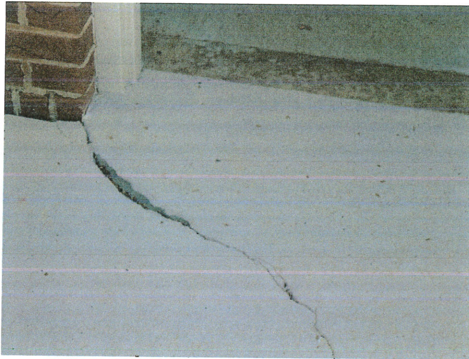
Photo #6 Pool deck condition
